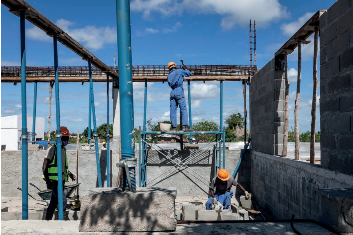
Resilient houses are built in the new Mutua neighborhood, Dondo District, Sofala Province. The project is part of the United Nations Development Program's Reconstruction Mechanism in support of the Government of Mozambique's actions for recovery after cyclones Idai and Kenneth in 2019. UN Mozambique/Chris Huby
