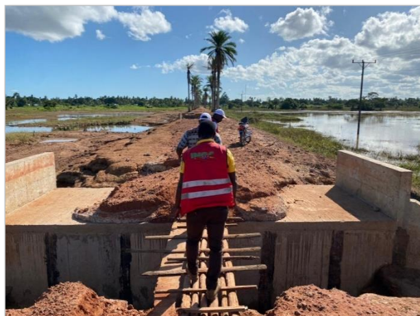
Figure 1: a damaged road in Maganja da Costa (Credit: RCO)
