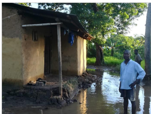
Figure 1: a damaged house built with adobe in Maganja da Costa (Credit: RCO)
