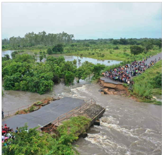
Figure 2: Interrupted EN1 road, between Nicoadala-Mocuba (Credit: INGD)
