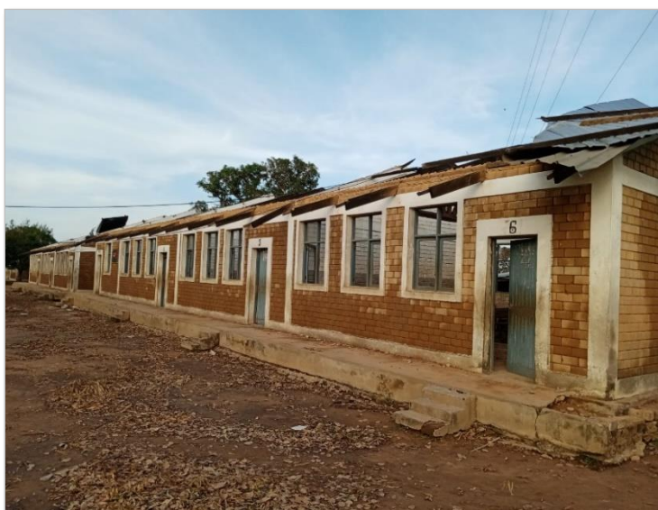
Figure 1: a damaged school in Mossuril. Credit: UNICEF
