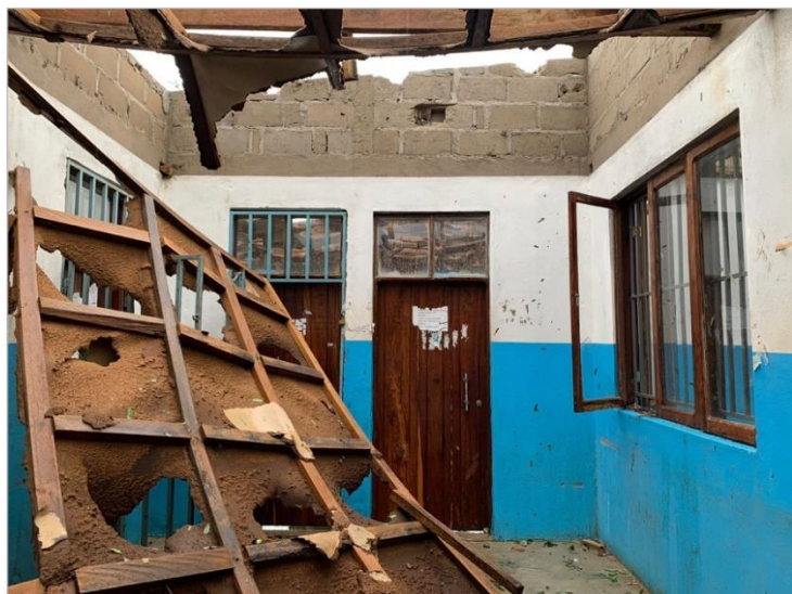
Damaged health center, Monapo District (UNHCR)
